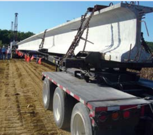
Beams were cast at Lafarge North America's plant in Winnipeg and trucked to the site.
